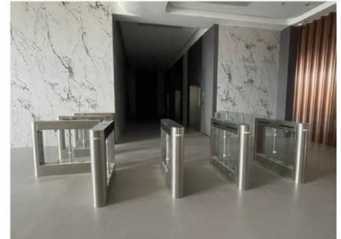
TAP CARD ELEVATOR
